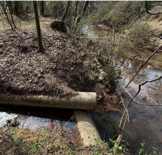
Eroded Creek Bank
