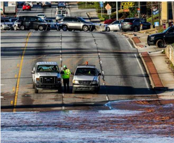
Buford Hwy Water Main Break
