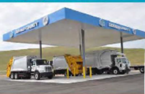
CNG Station - Seminole Road Landfill
