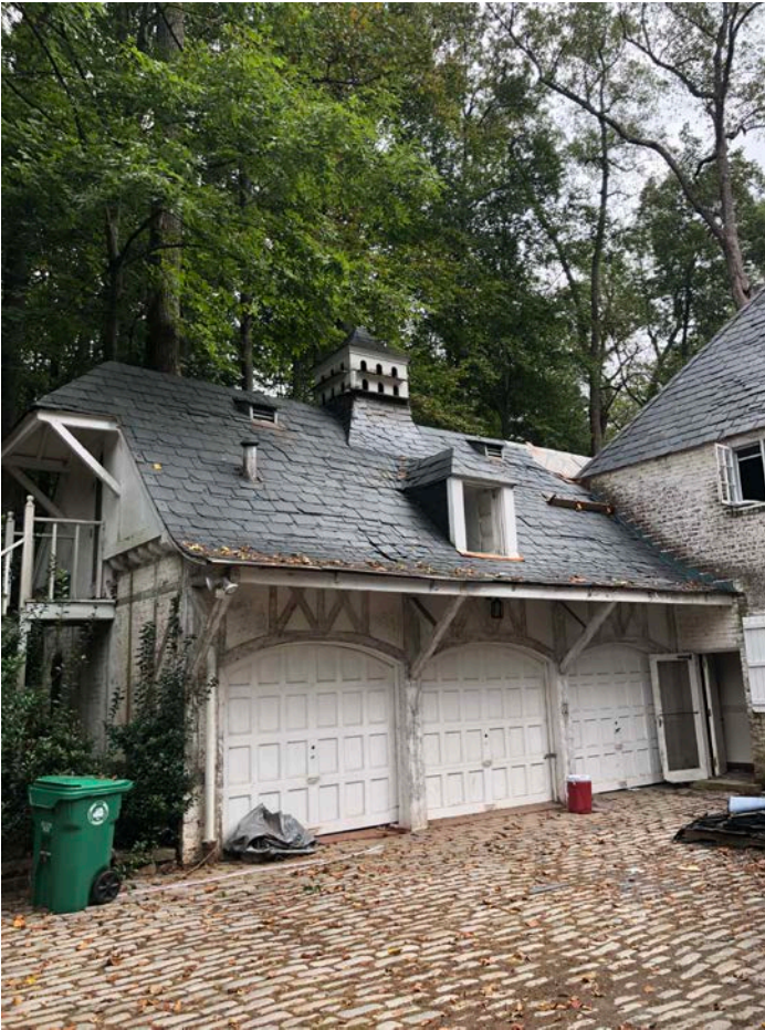
Supporting Pictures for item #3 - Demolish and rebuild the entire 3 car garage
