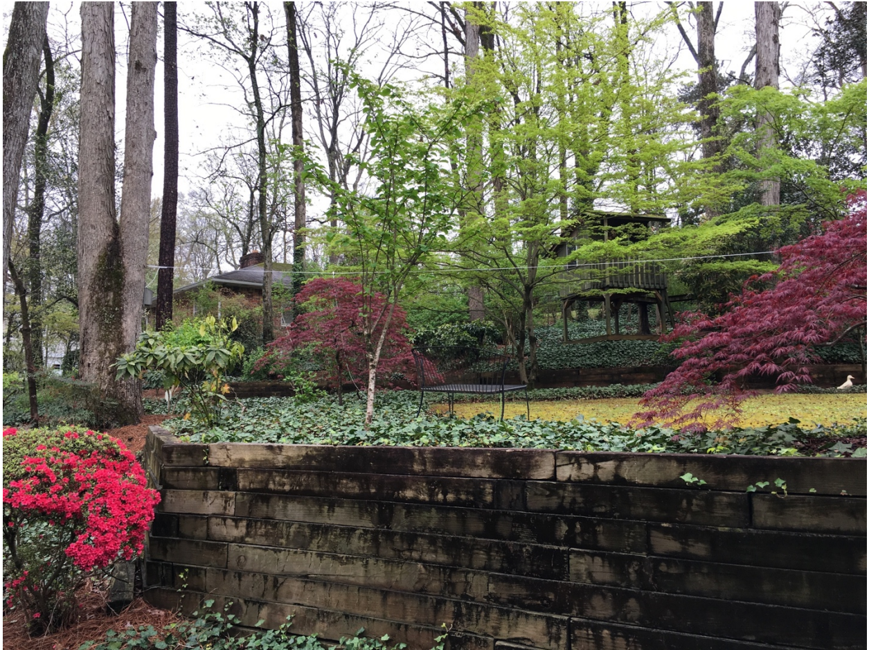
Photo 5: Looking south-east along north-east property line (property line is on the left side of photograph). Proposed Aluminum fence will be installed along existing wooden wall.
