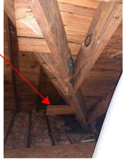
Photo 15 Dislodged Roof Rafter
