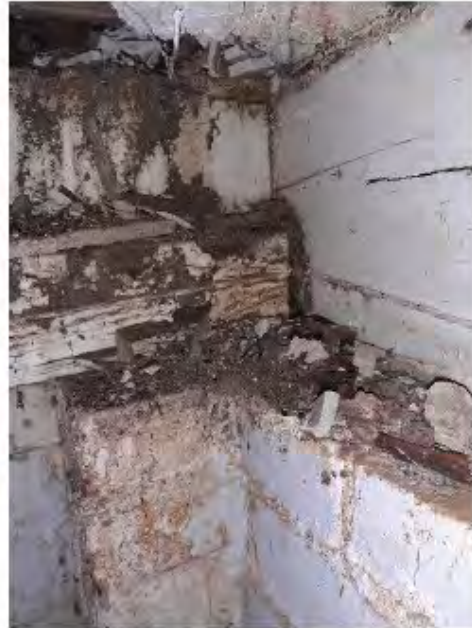
Photo 11 Water Leak Staining / Damage
