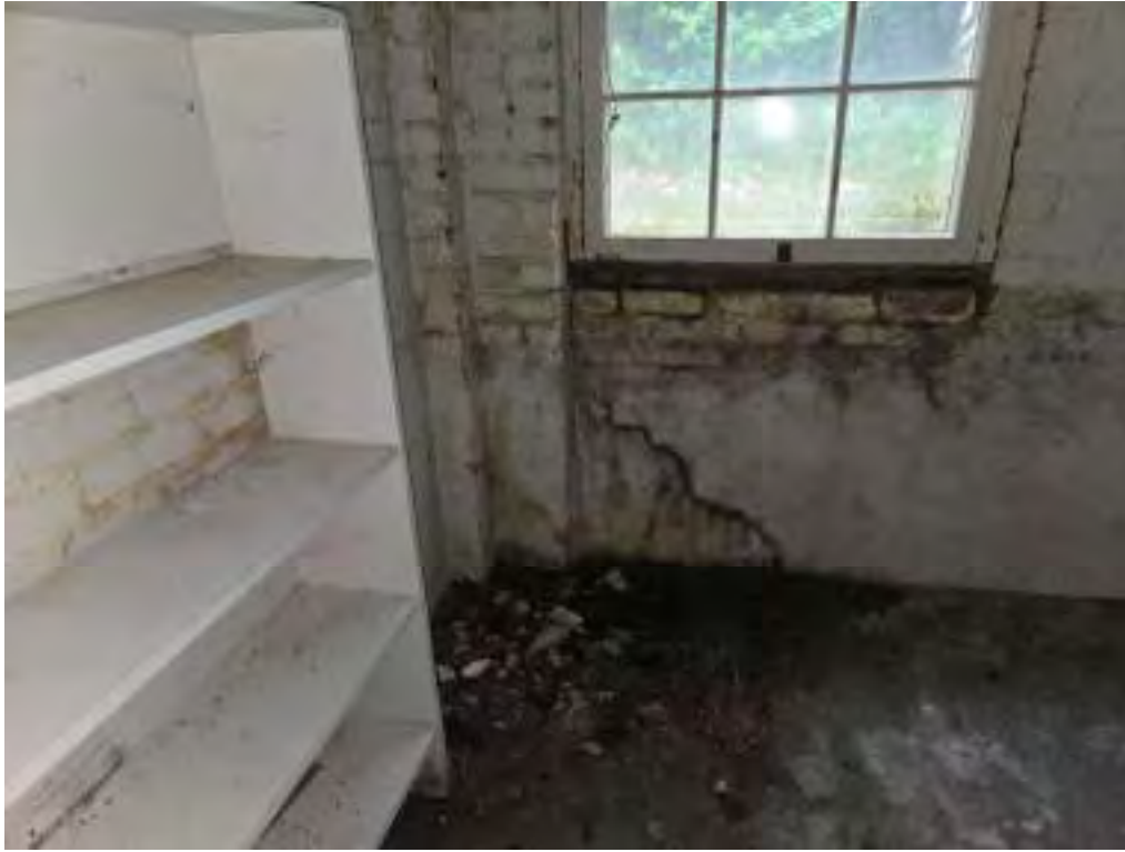
Photo 31 Cracked Northwest Exterior Foundation Wall Below Sunroom
