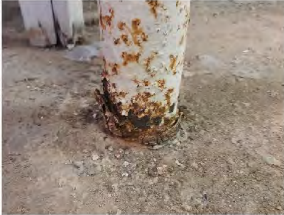
Photo 31 Rusted Bottom of Column
