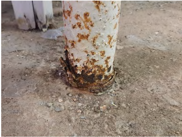
Photo 31 Rusted Bottom of Column
