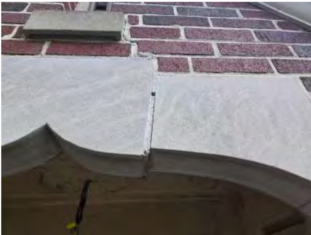
Photo 14 Entry Door Vestibule With Dropped Stone Pediment and Cracked Jointing
