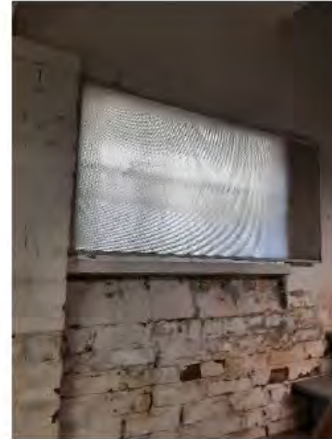
Photo 12 Water Leak Staining / Damage
