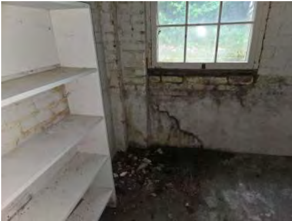
Photo 31 Cracked Northwest Exterior Foundation Wall Below Sunroom
