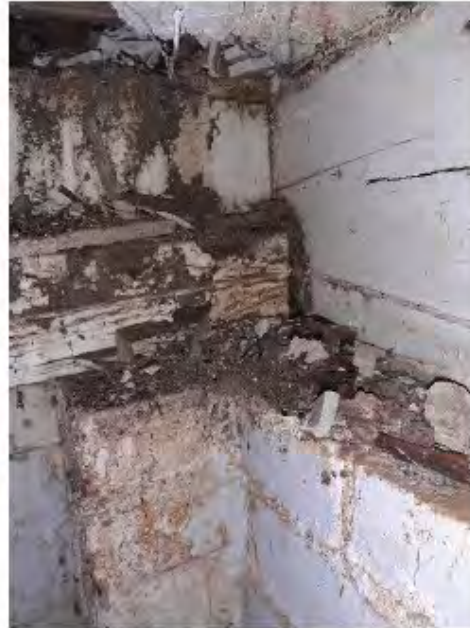
Photo 11 Water Leak Staining / Damage
