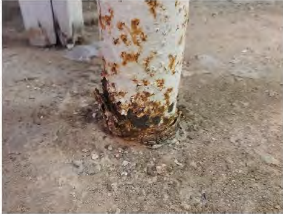
Photo 31 Rusted Bottom of Column
