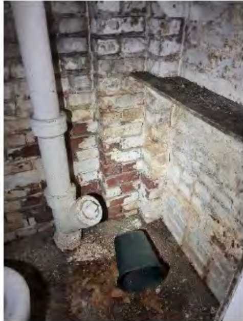
Photo 10 Water Leak Staining / Damage
