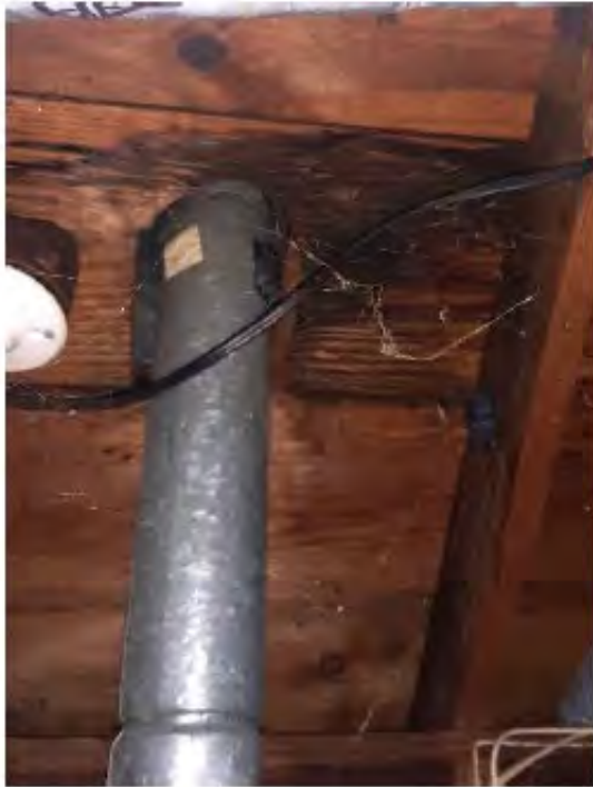
Photo 13 Water Damage at Vent
