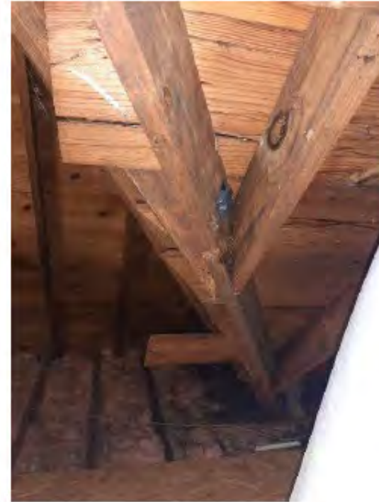
Photo 15 Dislodged Roof Rafter
