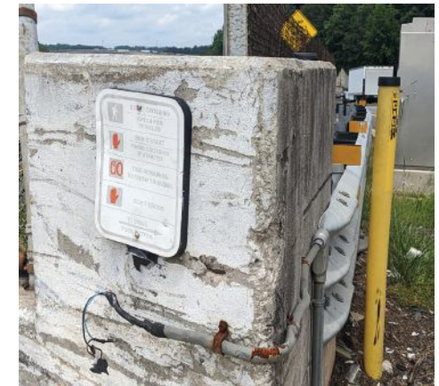
FIGURE 26 - BROKEN CROSSING INFRASTRUCTURE
