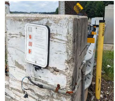
FIGURE 26 - BROKEN LIGHTED CROSSING INFRASTRUCTURE
