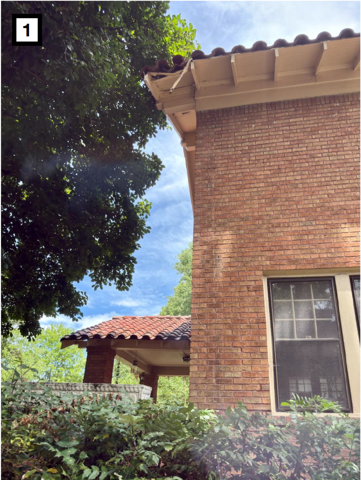
Location of damaged roof section, missing gutters & downspouts at northwest (front) corner of structure
