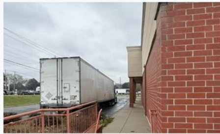
Photo 3: Deteriorating building facade
