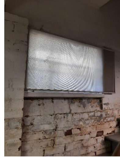
Photo 12 Water Leak Staining / Damage
