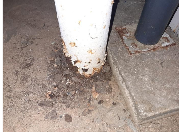
Photo 32 Rusted Bottom of Column at Adjacent Shoring Post
