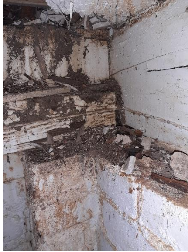
Photo 11 Water Leak Staining / Damage
