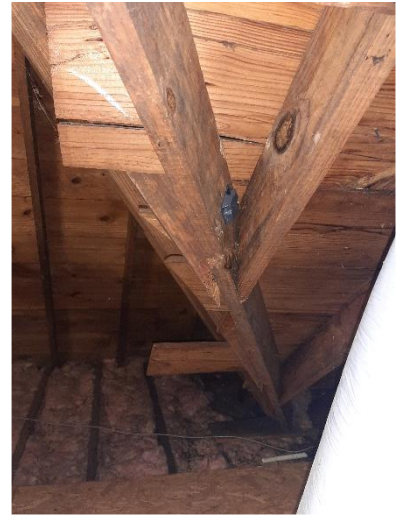
Photo 15 Dislodged Roof Rafter
