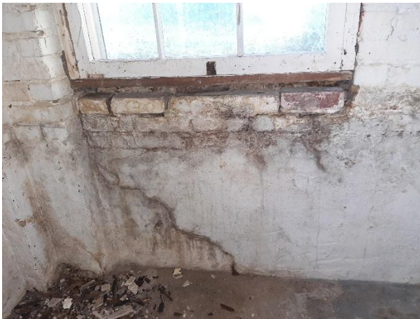
Photo 8 Stair-Step Crack at Basement
