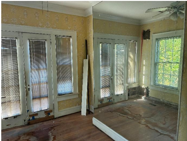
Photo 46 Water Damage at Floor of Sunroom / Enclosed Porch
