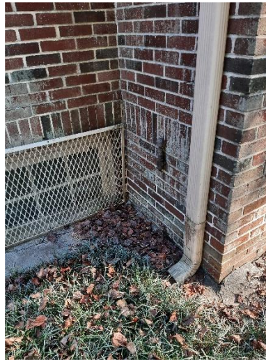
Downspout Near Basement Window
