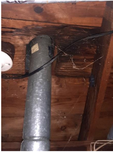
Photo 13 Water Damage at Vent
