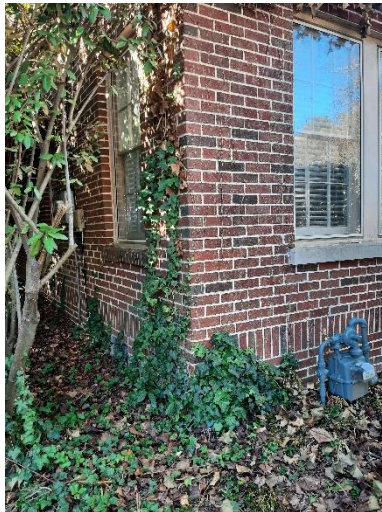
Photo 6 Stair-Step Cracks (SE Corner)
