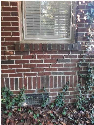
Photo 5 Stair-Step Crack (South Wall)
