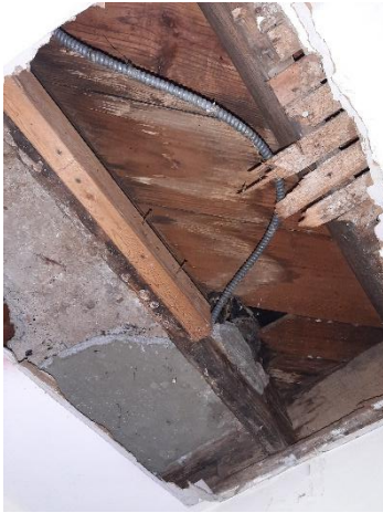
Photo 16 Damage at 2nd Floor Framing
