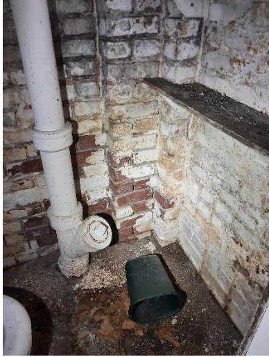
Photo 10 Water Leak Staining / Damage
