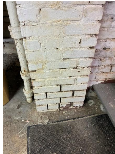
Photo 9 Loss of Mortar at Brick
