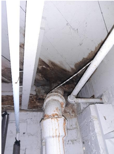
Photo 26 Floor Damage below Breakfast Nook
