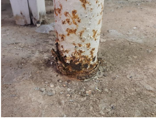
Photo 31 Rusted Bottom of Column
