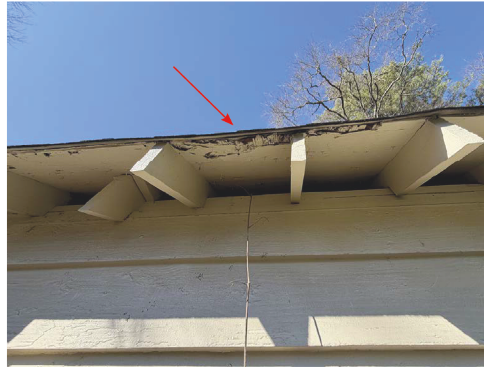
Sheathing rot. Significantly warped roof line.
