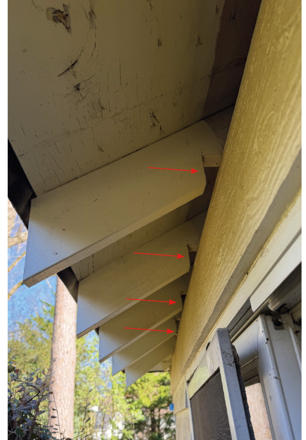
Roof joists not bearing on exterior stud wall due to differential settlement of foundation
