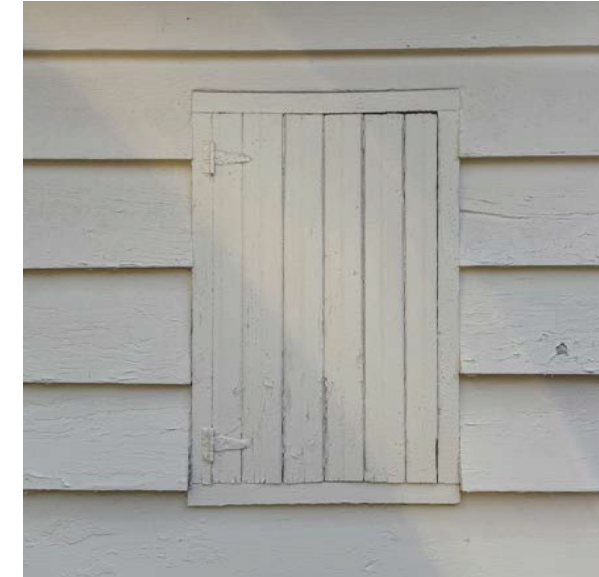
Wall openings: Similar type and dimensions to existing solid, vertical tongue and groove window hatches.
