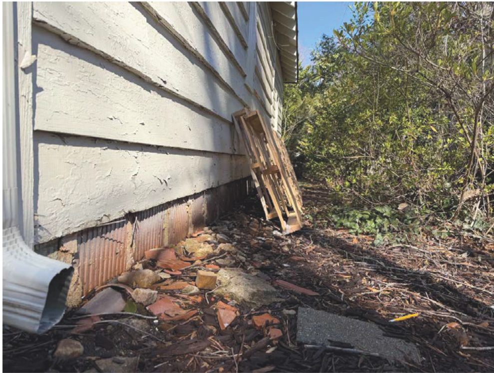
Spalling terracotta block foundation
