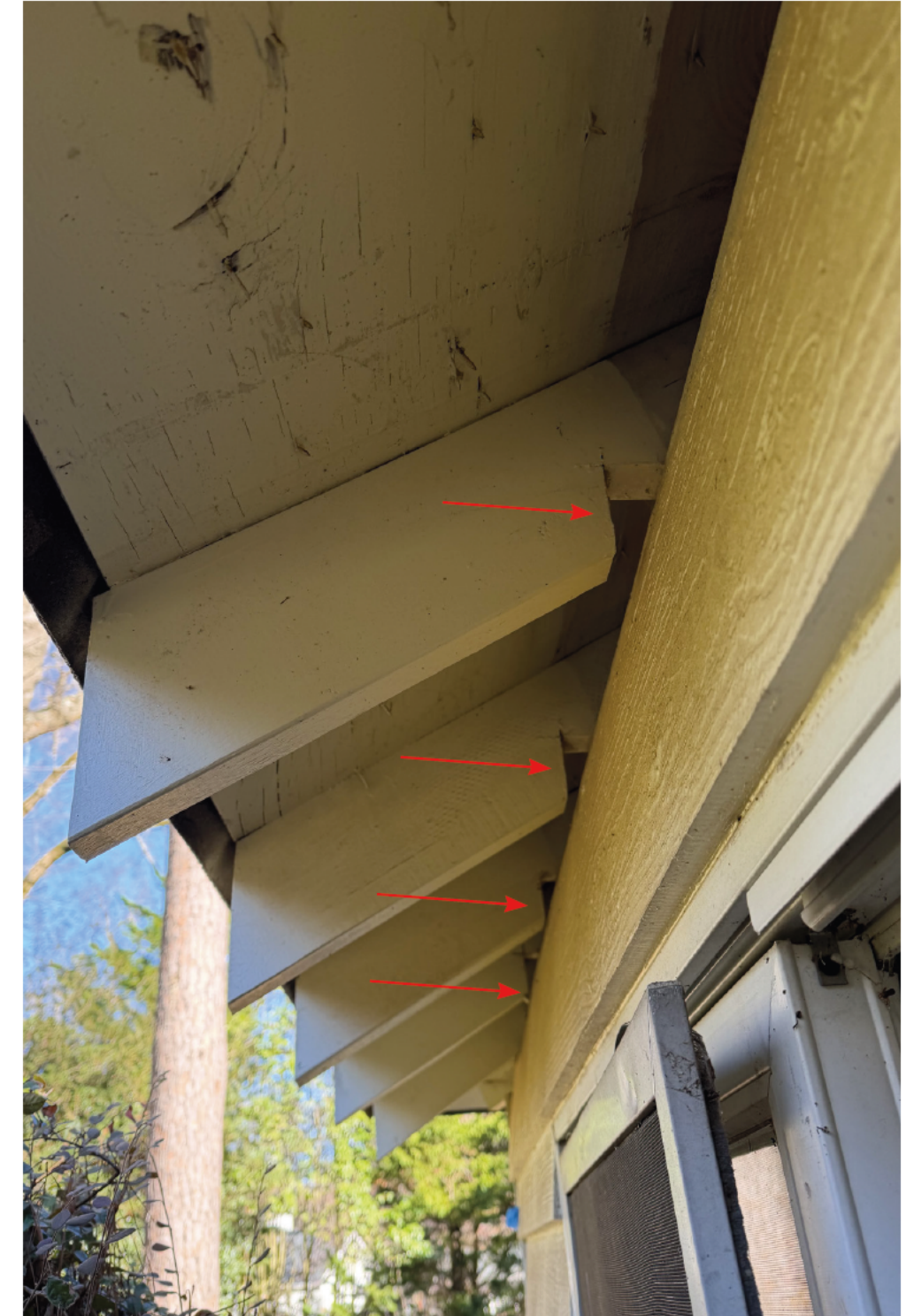
Roof joists not bearing on exterior stud wall due to differential settlement of foundation
