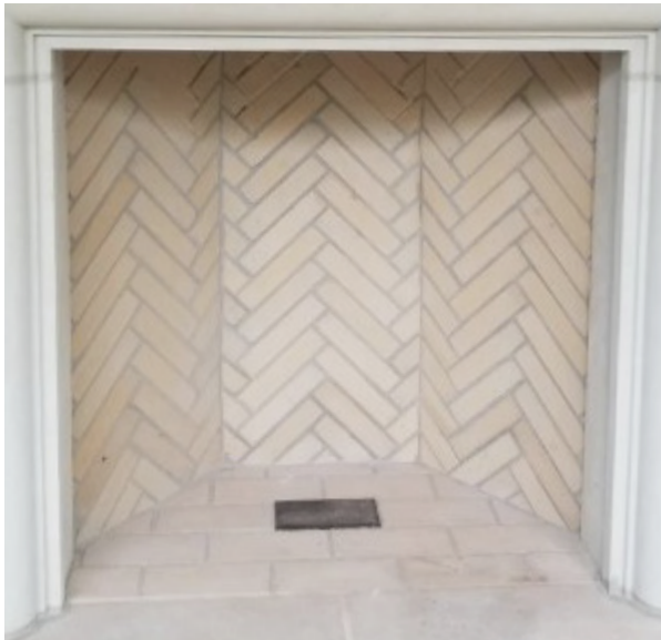
Fireplace: Isokern firebox with her- ringbone face fire bricks
