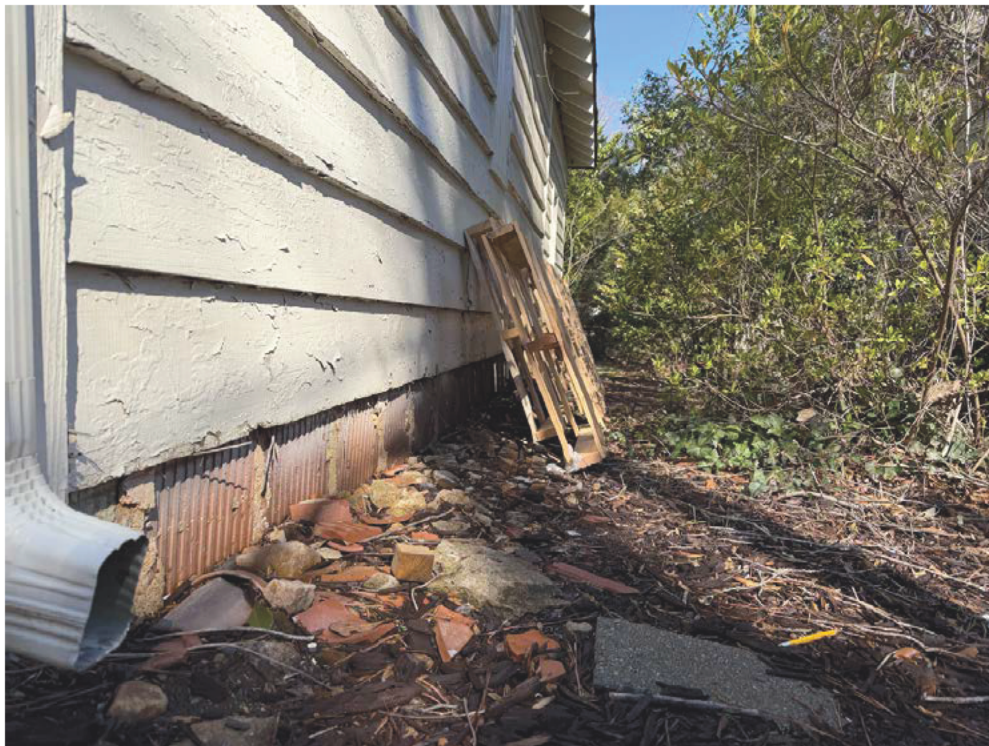
Spalling terracotta block foundation
