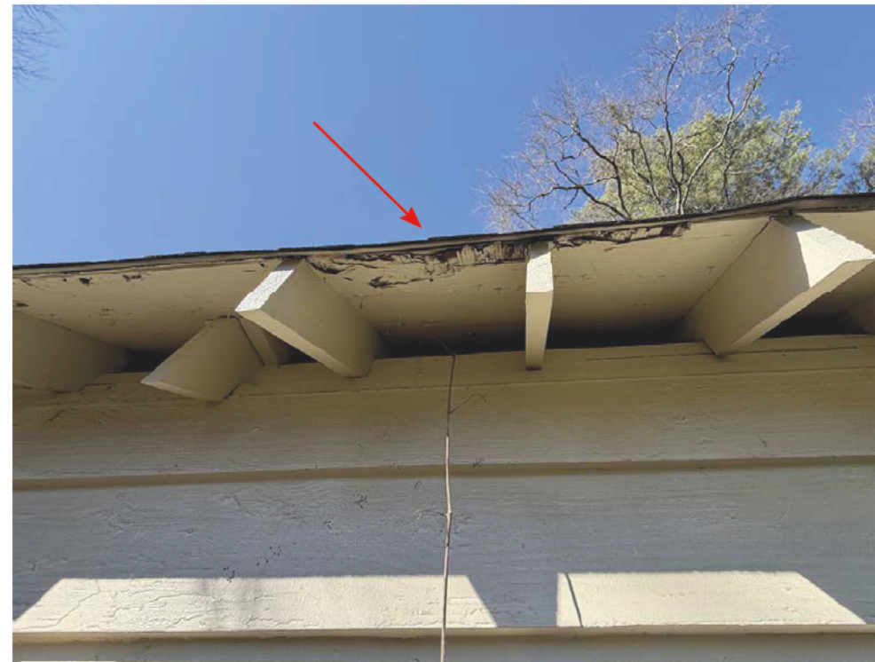
Sheathing rot. Significantly warped roof line.
