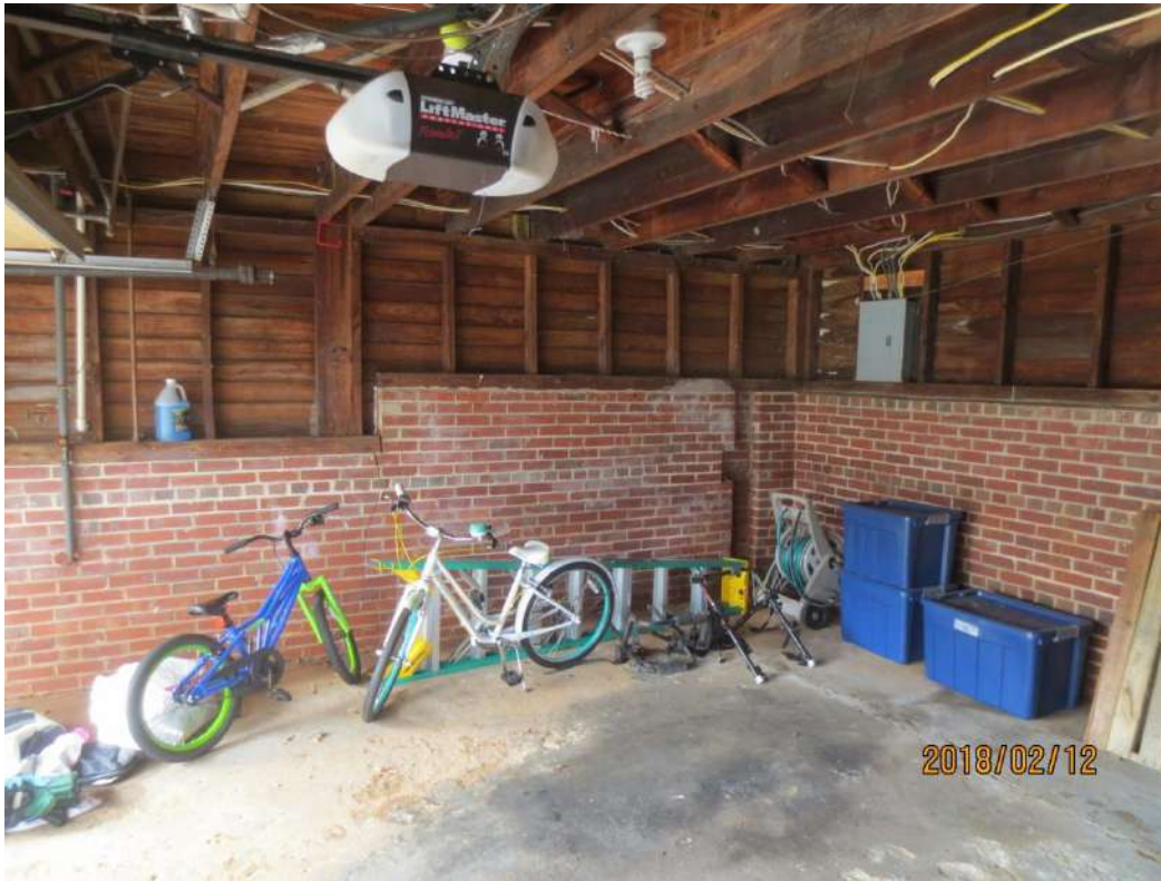
Left foundation wall and over-spanned 2x12 joists
