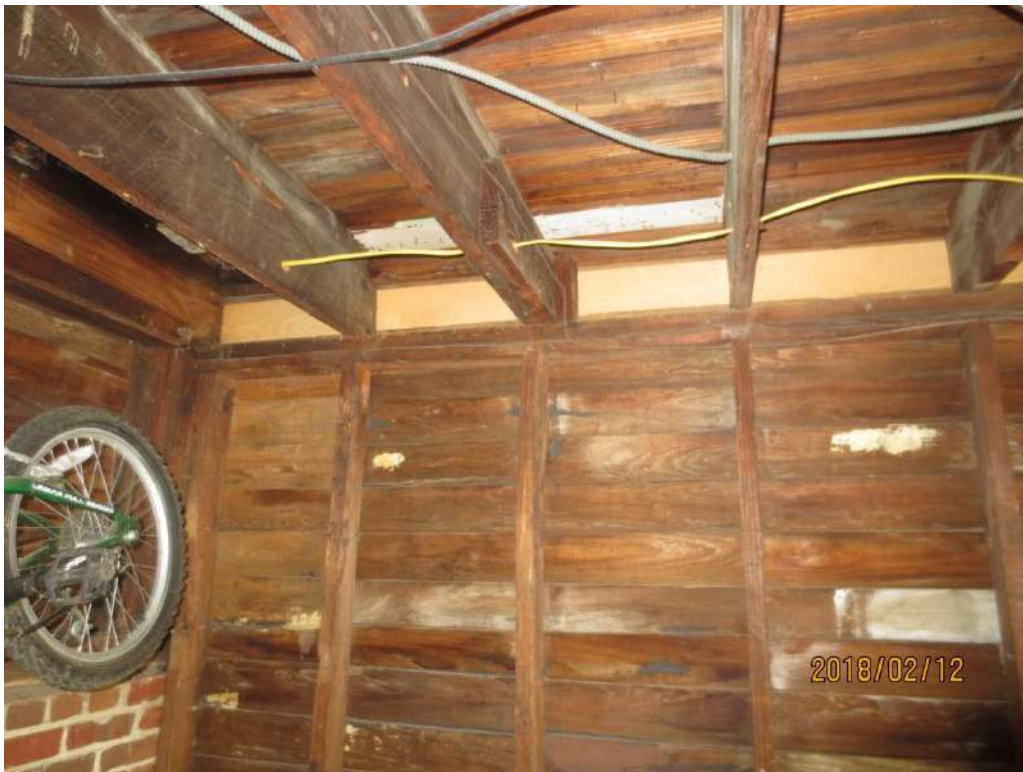
Damaged wall framing to be replaced
