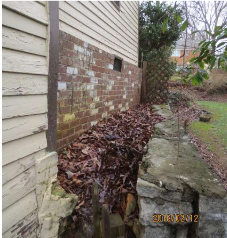
Addition side wall to be replaced
