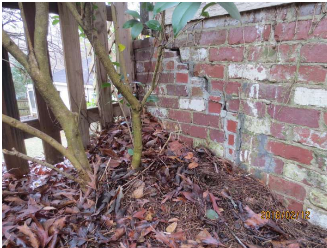
Rear addition corner settlement to be re-built with new footing and wall
