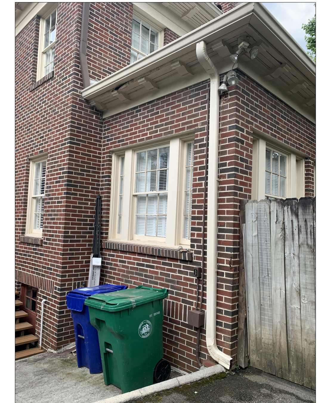
CONCRETE LANDING SLOPES TOWARDS BASEMENT WINDOW
