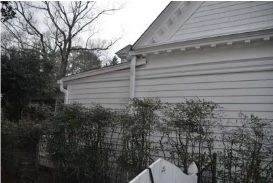
6. VIEW OF SIDE where proposed changes involve introducing windows and replacing non-historic siding with cementitious shingles & pilasters
