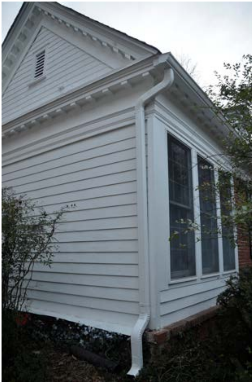
4. VIEW OF FRONT & SIDE where new windows and flat pilasters are proposed
