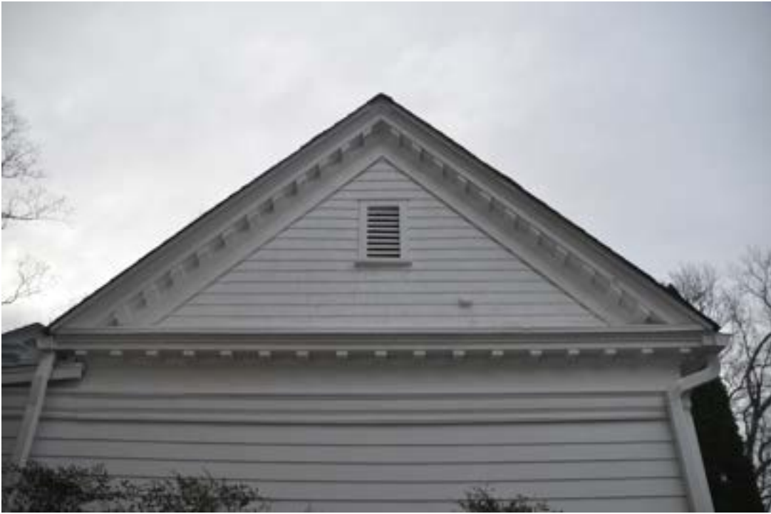
5. VIEW OF SIDE GABLE where original cornice, gable trim, louver & wood shingles will be retained
