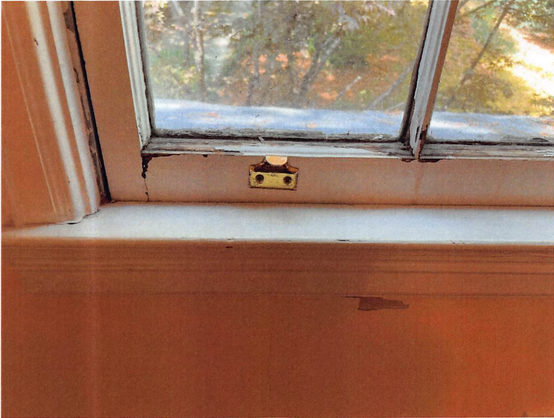
Figure 11: Window sash rot from condensation water damage
