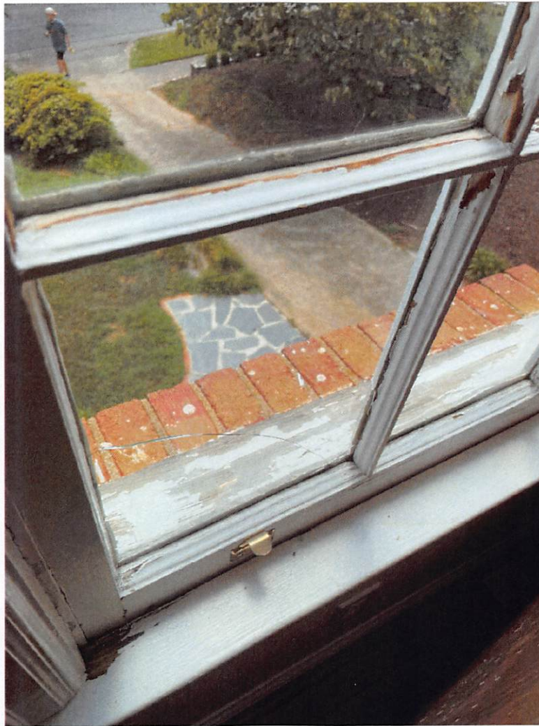
Figure 9: Cracked windowpane at front dormer
