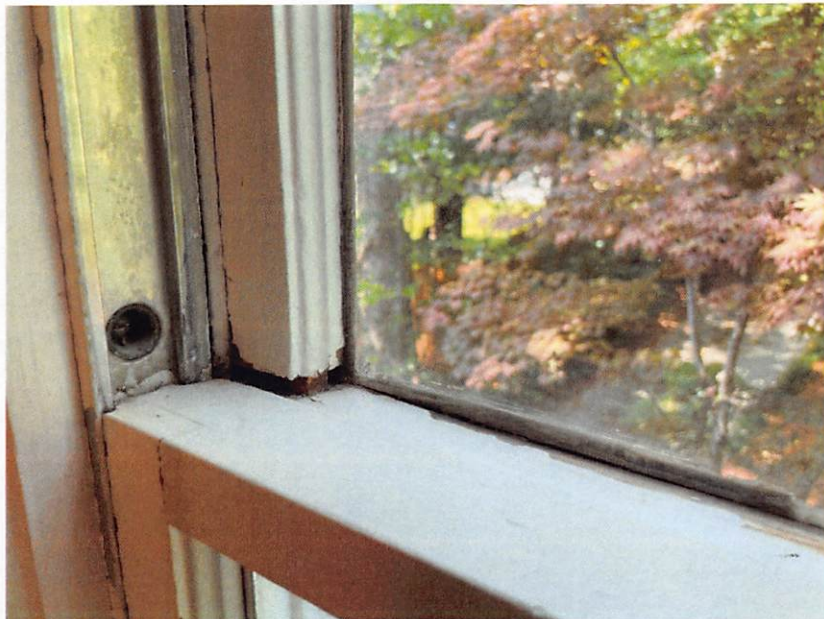
Figure 10: Window sash rot from condensation water damage
