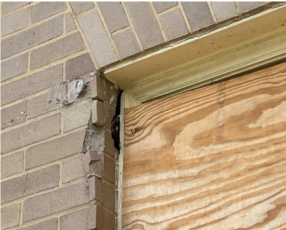
IMG EX6-3: Crumbling wood on the top corner of a jack arched window.
