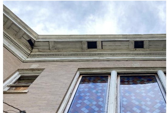
IMG EX6-4: Deteriorating roof trim on west side of mansion.
