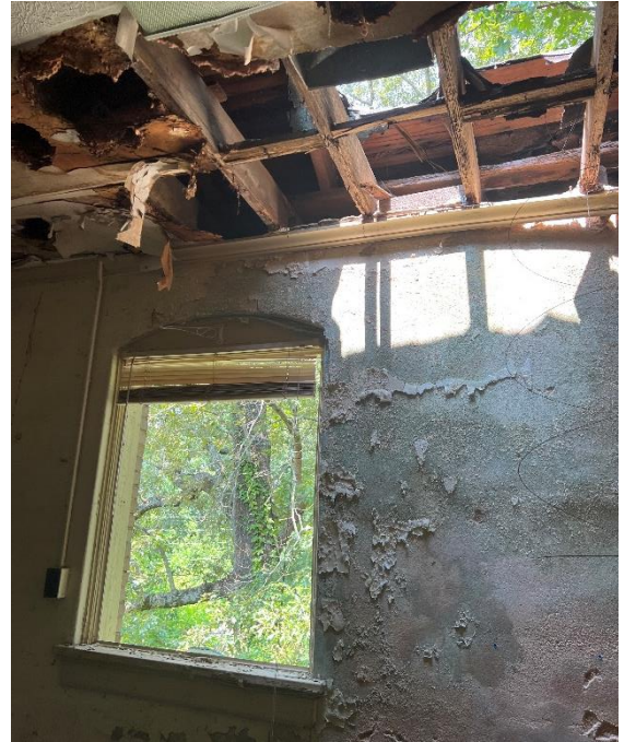
IMG CH3-2: Hole, one of two, in roof allowing structural deterioration. Framing repairs needed before roof replacement.
