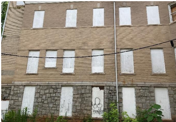
IMG EX2-3: Boarded up windows cover the East Wing of the Candler Mansion, largely protecting the broken windows that lie behind.
