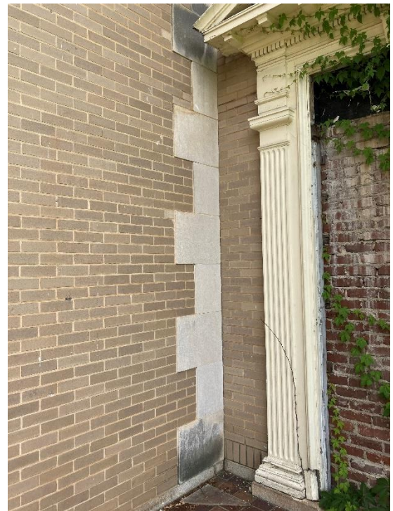
IMG EX5-5: Corner of entry patio containing many typical materials used extensively around the Candler Mansion.
