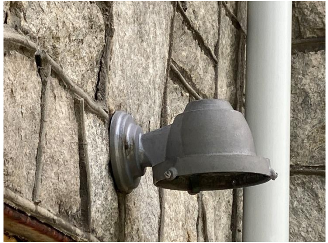
IMG CH2-2: Close up of stone on Carriage House with fixture and pipe running along. Original fixtures are going to be maintained in restoration.
