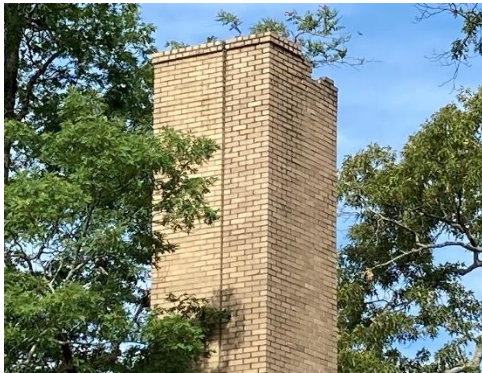
IMG CH3-3: Replacement needed on chimney with bricks missing on the top.
