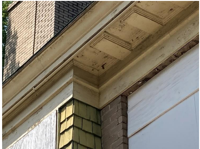
IMG CH2-4: Corner where deteriorating paneling connects with trim as well as brick wall.
