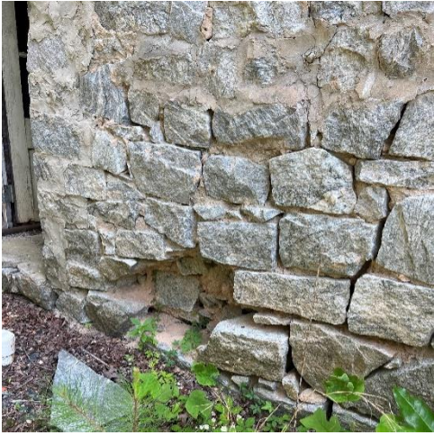
IMG CH3-1: Missing and cracked stone on basement level.
