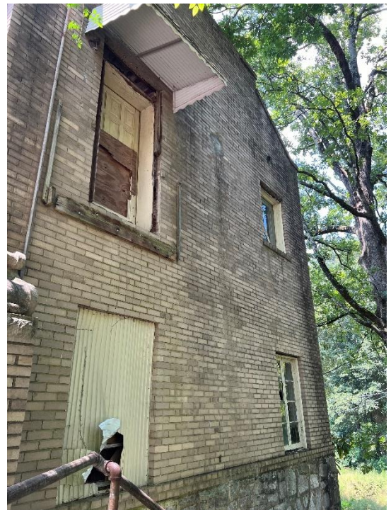
IMG CH1-2: North side with stairway down to back of Carriage House. Replace door with window matching adjacent.
