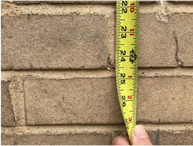
IMG CH2-1: Typical size of brick in both the Main House and Carriage House.
