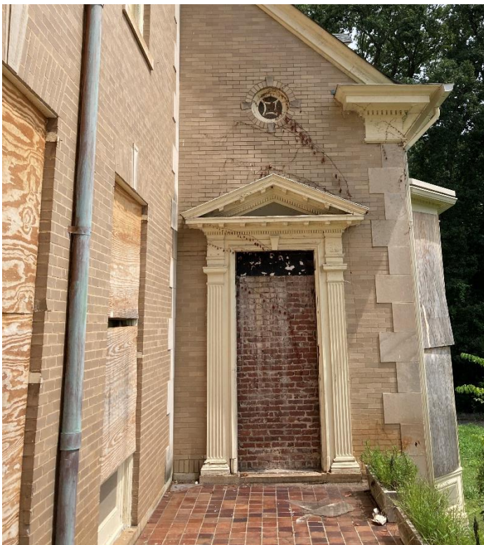
IMG EX4-3: Detailed trim of brick-filled door that leads to nothing on the interior side. Trim needs repair.
