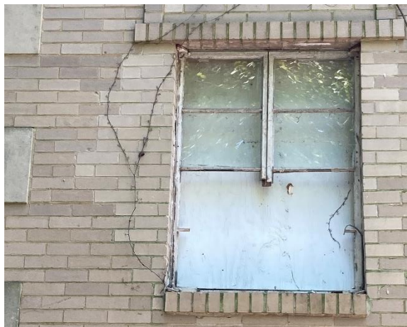
IMG EX6-5: Broken steel window on the Organ Room; typical for many steel and wood windows around the property.
