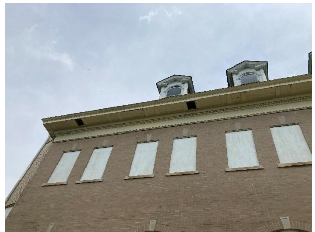
IMG EX3-4: Jack arch windows in the children's rooms above the Solarium. Brick on Southeast side is largely in good condition.
