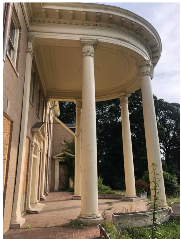
IMG EX4-4: Entry patio for main door. Column bases need to be addressed.
