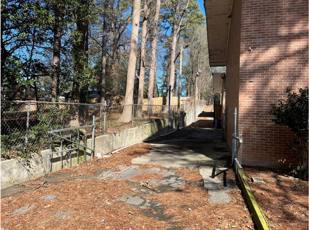
Existing west side elevation, as seen from the driveway at the back of the buildings:
