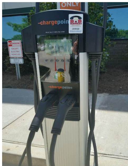
The station located at 3720 Leroy Scott Drive is one of two others B&B Services Electrical & Communications installed (MORE)
